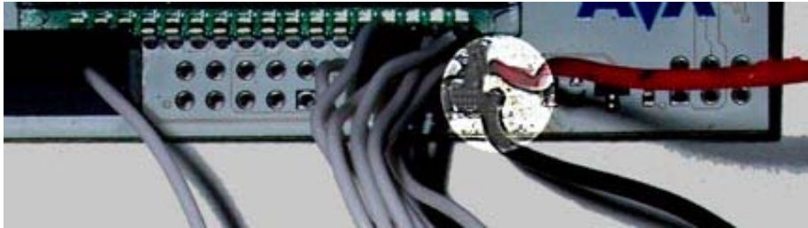
Figure 5: External battery connection to Butterfly
